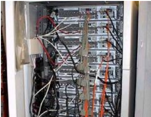
Rack Mount Server
